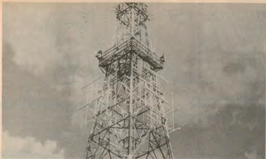
Most TV antennas are variations on the basic dipole antenna as described in this article. This large array is for Channel 0 in Sydney. The large dipoles can be easily recognised, ie, the hefty lengths of horizontal pipe painted white.
