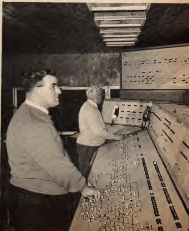
Part of the control panel in Rugby signal box, from which remote interlockings are operated by an electronic supervisory system
