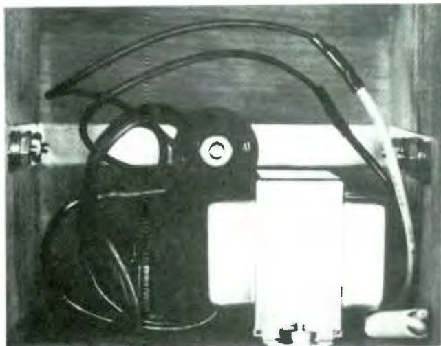
Shown here is the circuit mounted and ready to operate. Note the large air space around the magnetic coil. That helps keep it cool. Do not use a cabinet that is too small.
