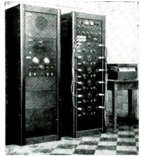
Six amplifiers are mounted in rack at right.
