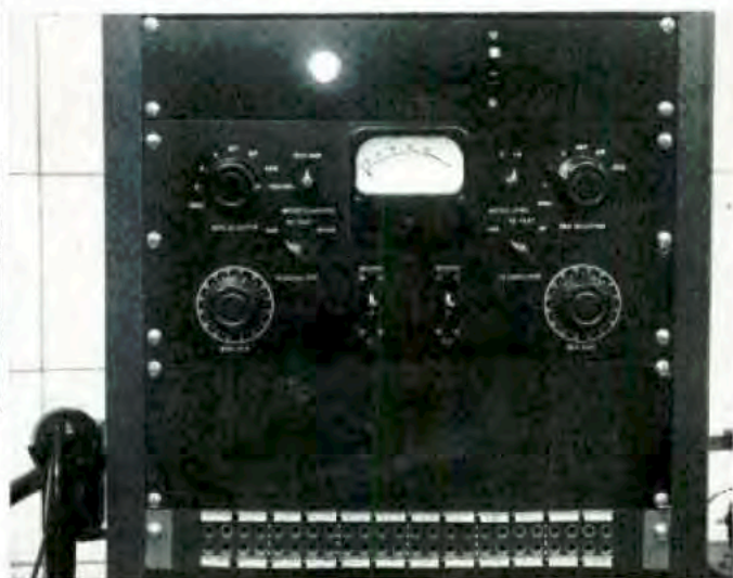
Fig. 7. Control panel and patch field of recording bay. All bays are identical.
