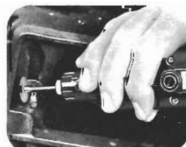
Cut off bolts
