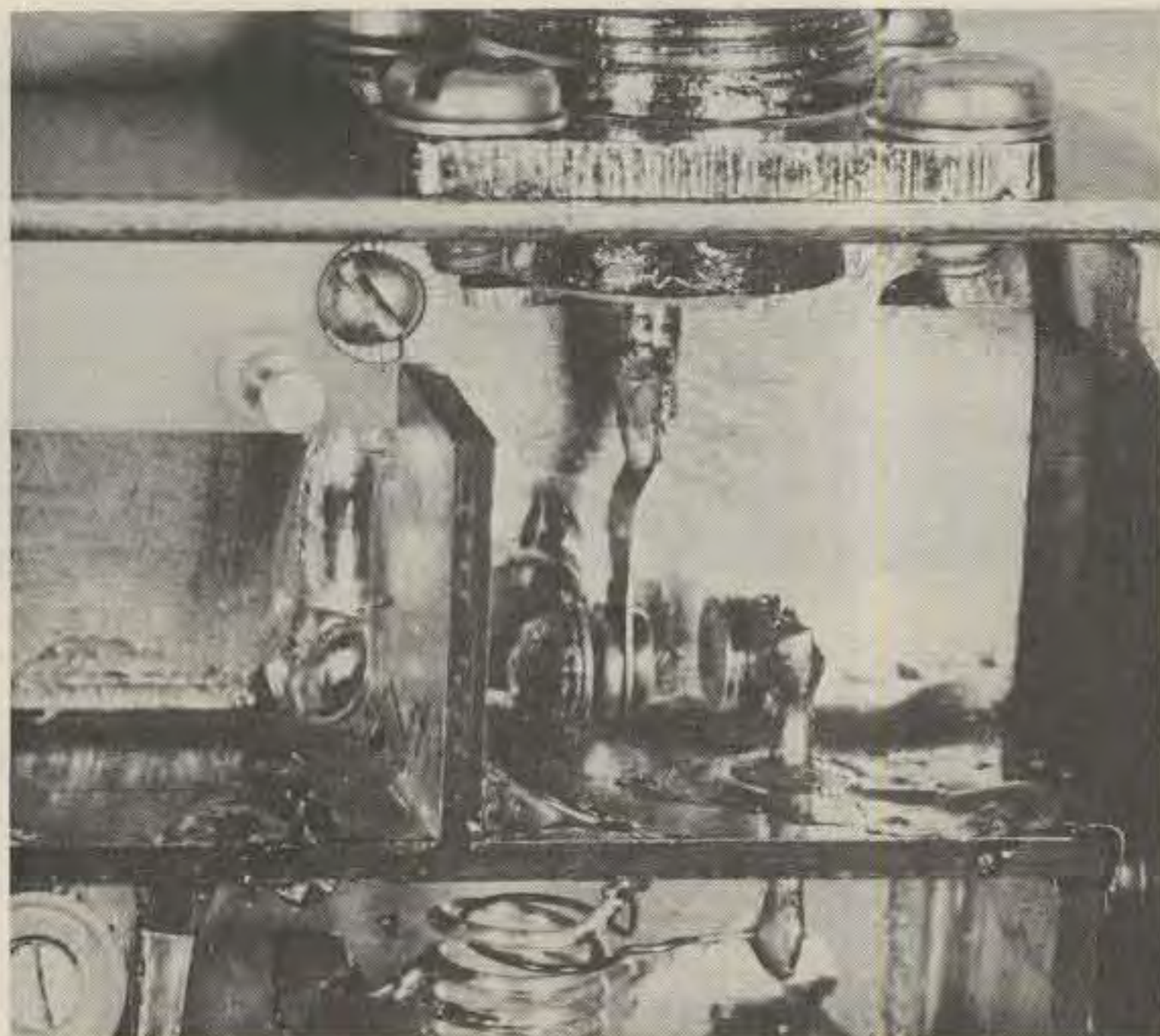
A detailed view of the input contacts of the preamp. The glass feedthroughs are visible, and the method of attaching the relay contacts to the feedthroughs can be seen.
