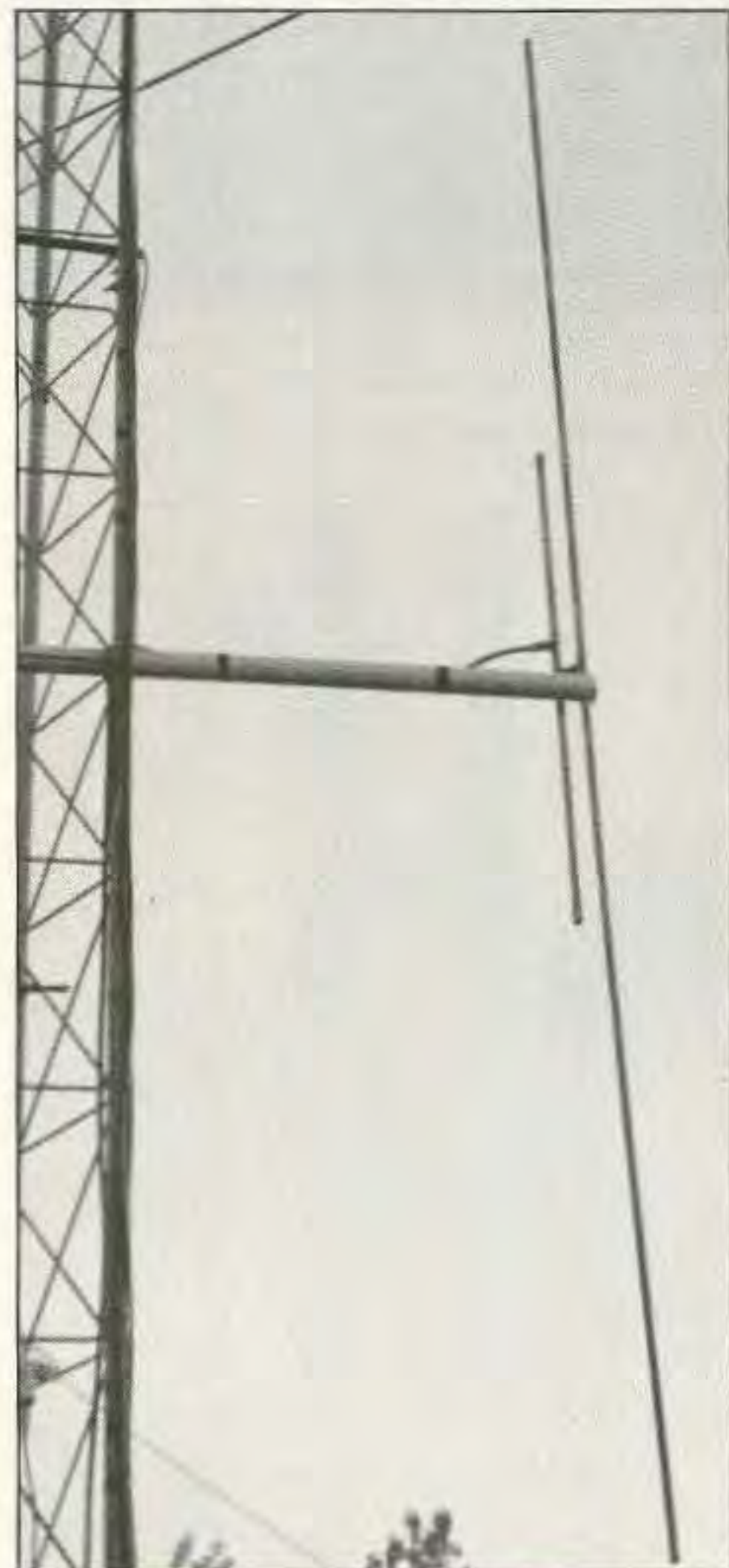
Photo C. Use PVC pipe to mount the Cactus to the side of your tower. The Double Cactus is shown here.
