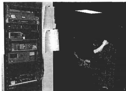
FIG. 3—A CONTROL ROOM OPERATOR INSPECTING broadcast equipment at KUSW, in Salt Lake City, UT.
