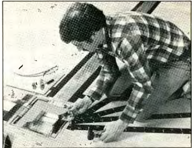
Technicians make a transition splice between a flat optical cable and a round optical cable in recessed floor junction box. The blanking tool, shown, provides a clean, precise square-off end of the optical fiber.
