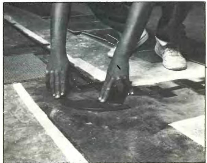
Carpet tiles, which completely conceal flat fiber-optic wiring, are usually held down with release-type adhesive to permit easy removal if outlets or wiring require rearranging. Fiber-optic cable does not require any special shielding or other protection.
