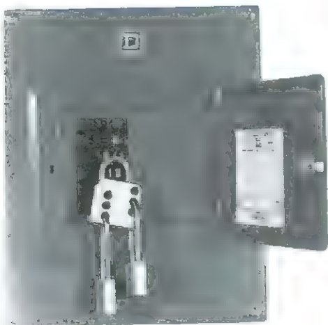
Figure 9.13 — Before working on a tower or antenna, disconnect and if possible lock out the ac power circuits for your radio equipment.
