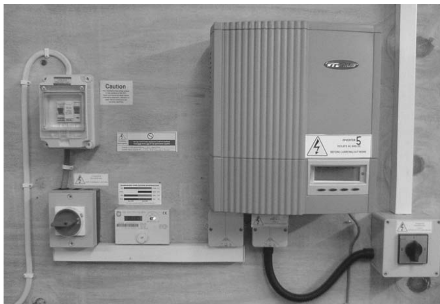
Figure 10-41 A typical inverter setup.
