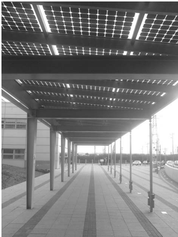
Figure 10-33 Bifacial solar cells on the roof of a covered walkway.
