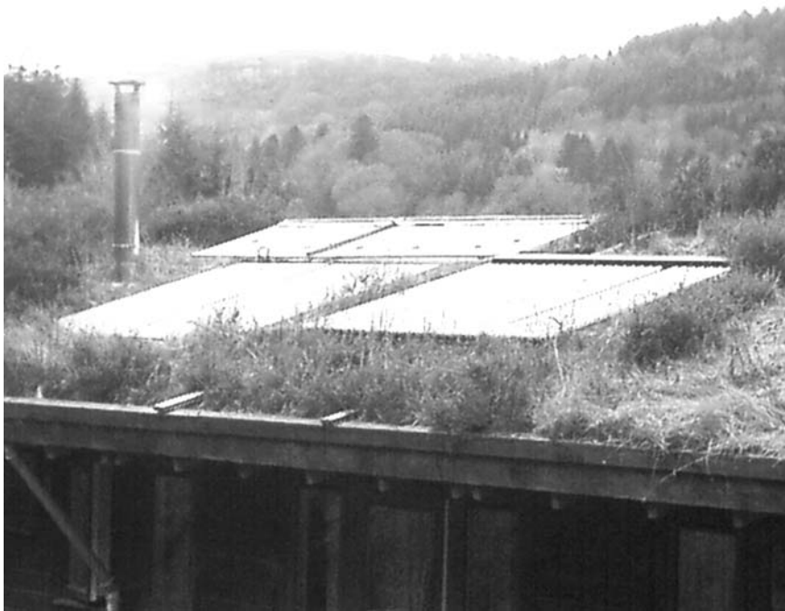
Figure 2-7 Solar energy being harnessed directly on the roofs of the eco-cabins at the Centre for Alternative Technology, U.K.
