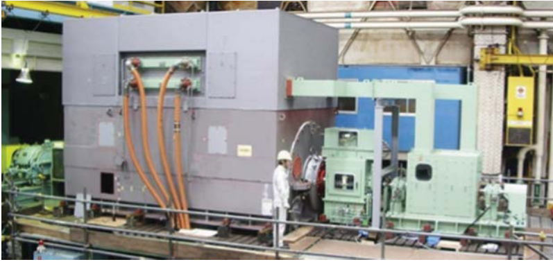
Figure 22.10 53 MW, 3000 rpm synchronous motor (Reproduced by permission of TMEIC)
