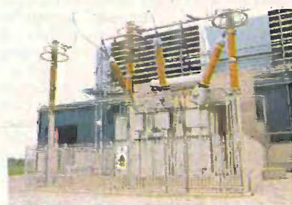
Four 400kV transformers connected to the outputs of the four generators.
