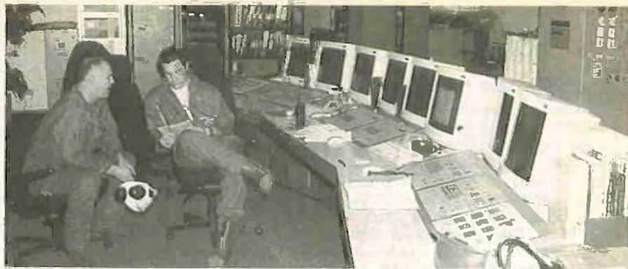
The computer control room monitors and records the performance of the plant.
