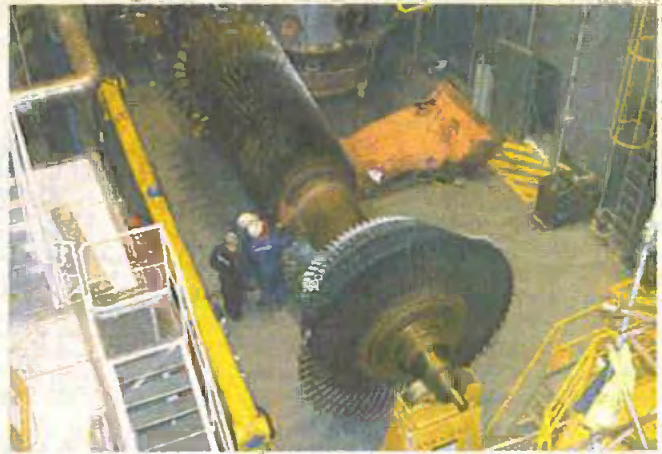
Aerial view showing gas turbine blades (largest, front) and air compressor (rear) on the shaft, undergoing inspection.
