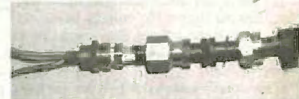
A typical armoured-cable terminator, note the steel armour which is the "protective earth".
