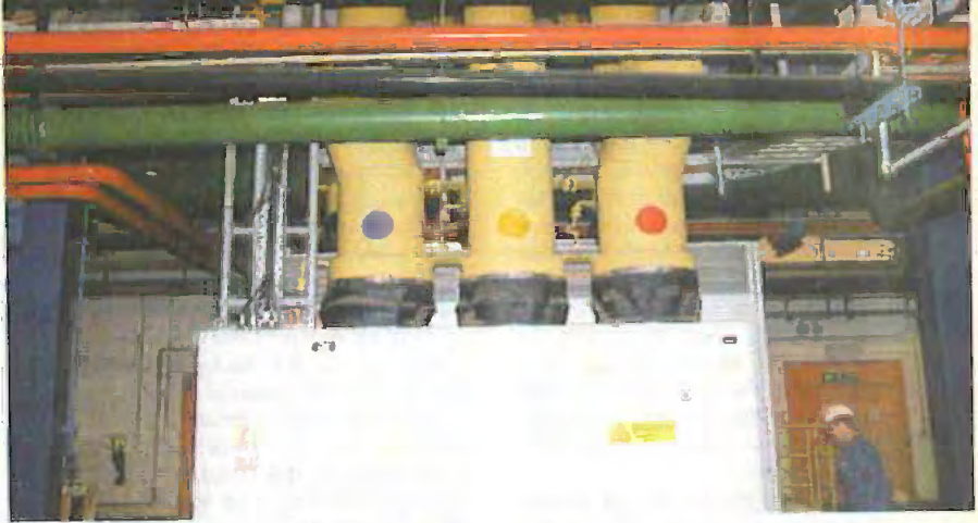
A circuit breaker unit connected to the gas turbine. Notice the colour coding "spots".
