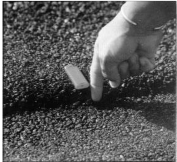
Figure 3.8. Overfilled patch area
