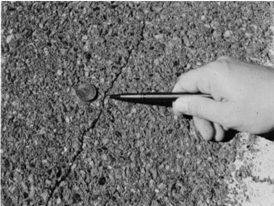
Figure 7.1. Example of hairline-size crack
