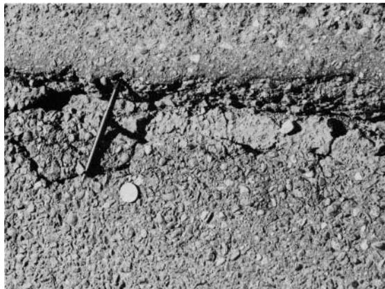
Figure 7.4. Example of large-size crack
