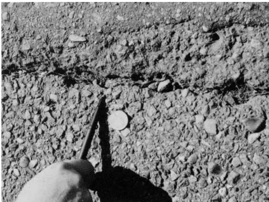
Figure 7.3. Example of a medium-size crack
