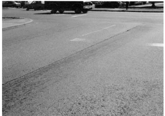
Figure 3.2. Example of longitudinal cracking
