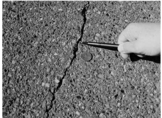
Figure 7.2. Example of a small-size crack
