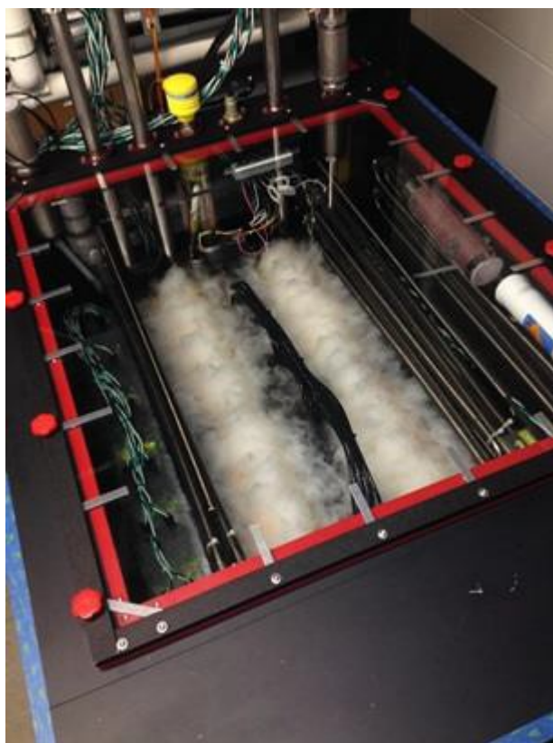
Figure 5-2: Pilot Test - IT Running at Full Power.
