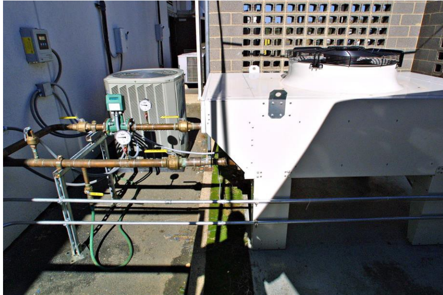
Figure 4-3: Dry Cooler Outside of NRL Data Center
