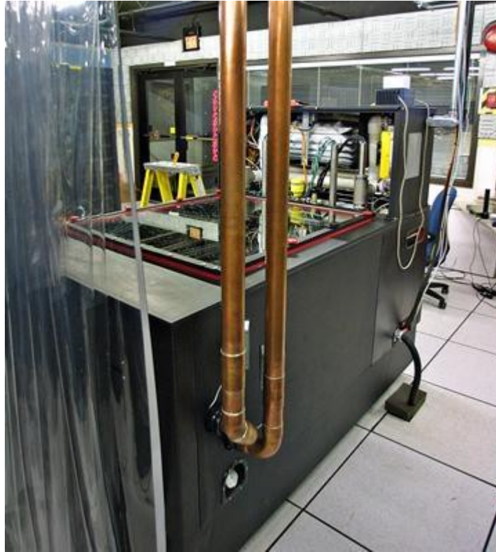
Figure 5-3: Immersion Case Test Installation (Demonstration)
