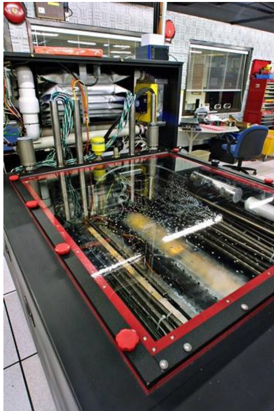
Figure 4-4: Bath Located in the NRL Data Center Room
