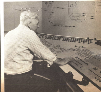
(below) Control panel of the "windowless" signal box at Leeds City station
