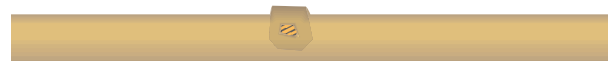
Figure 1. The insulation is pinched through to the conductor. The wire must be replaced.
