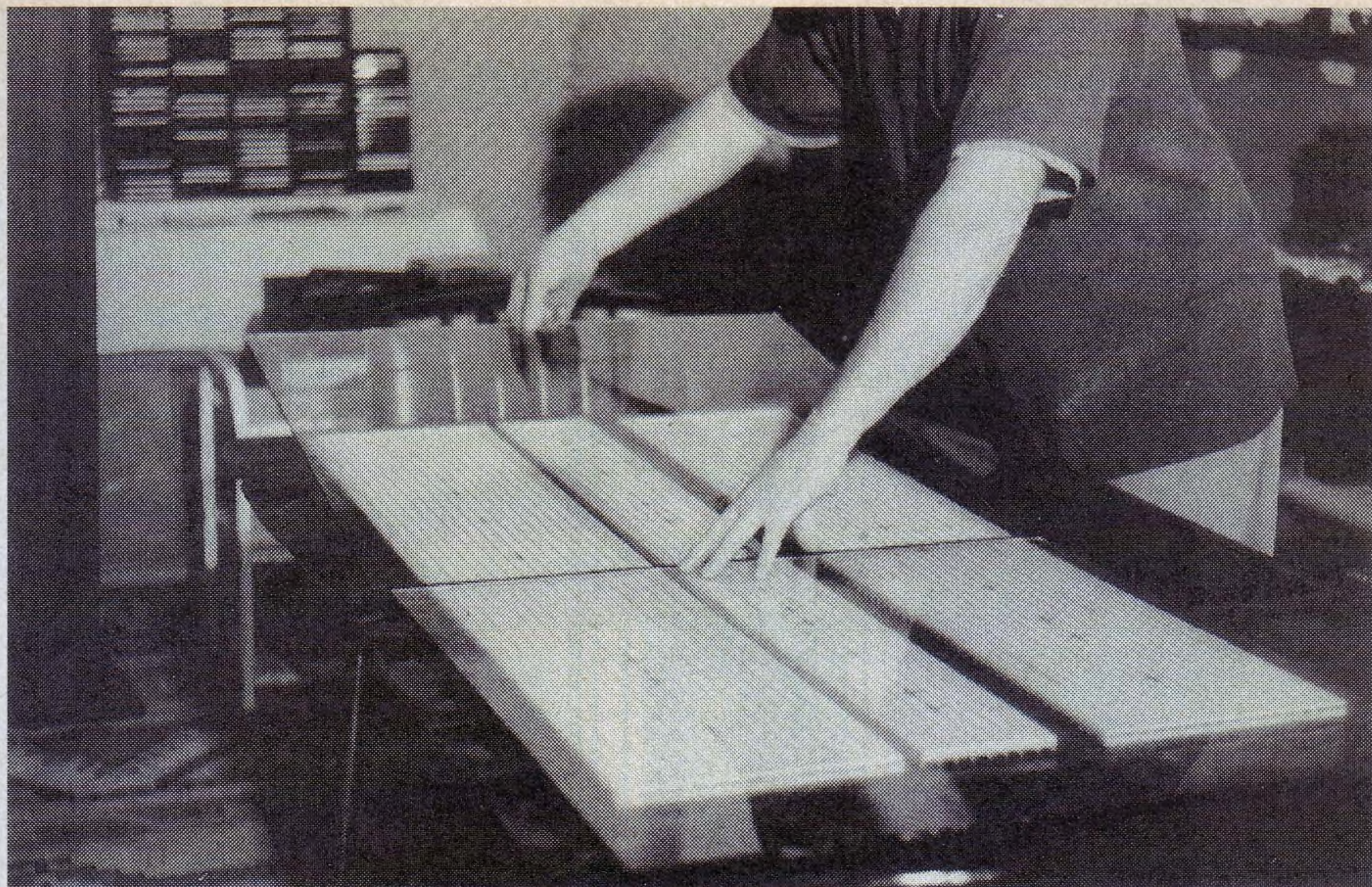
After the air gap spacers have been attached, pressure pads are applied while the adhesive sets. In this case, plate glass sheets are being placed and these will be weighted down with bricks.
