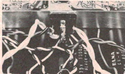
Mounting and wiring of the bridge rectifier. The + terminal is uppermost here.
